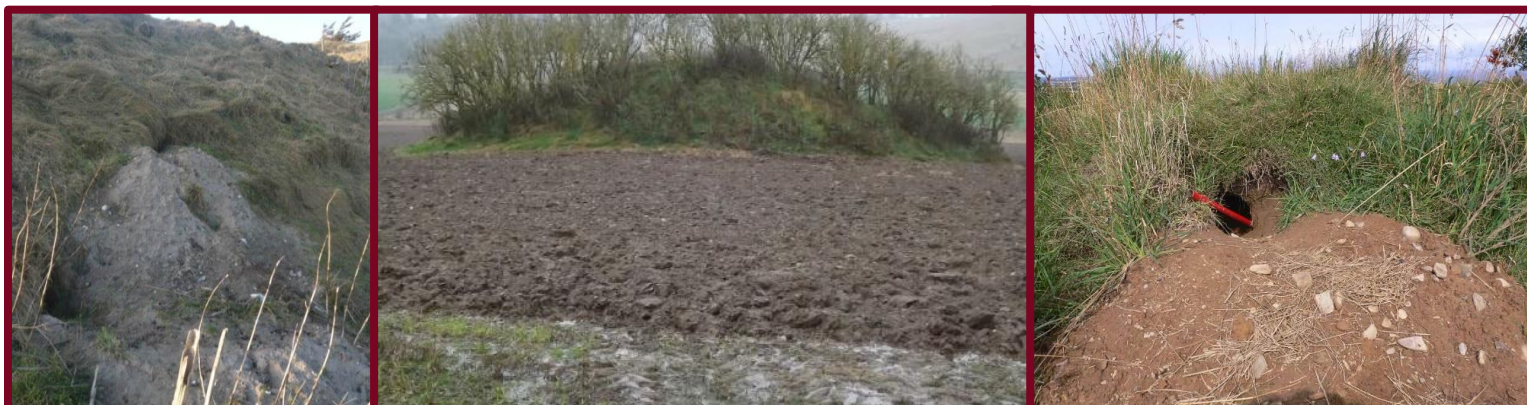
Burrowing animals, scrub and other vegetation can cause damage to scheduled monuments
